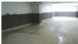
Town Hall, Kolkata: Successful Application of Convac Plus
