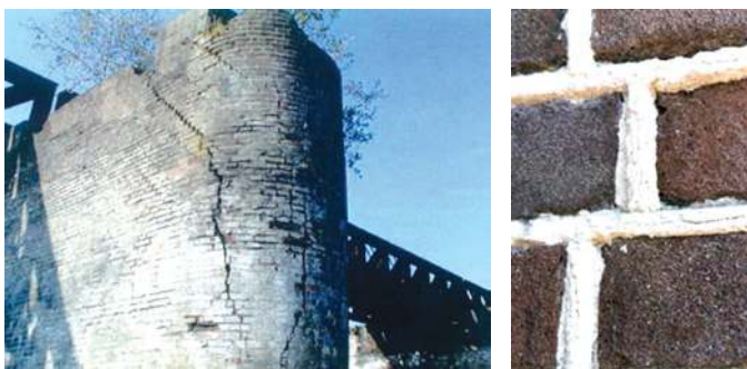
(a) Crack pattern in masonry, looking like structural damage but caused by expansive reaction in the internal part of the mortar; (b) Bursting of pointing mortar due to the formation of \text{CaO} \cdot \text{Al}_2\text{O}_3 \cdot 3\text{CaCl}_2 \cdot 31\text{H}_2\text{O} (trichloride).
