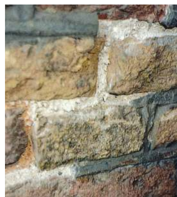
Push-out of cement re-pointing due to crystallization of salts at the interface of new pointing and old bedding mortar.
